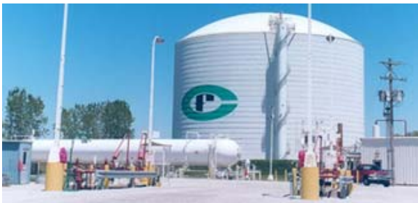
Fig. 7. “Atmospheric” refrigerated liquid anhydrous ammonia (NH 3 ) tank stores 190,000 MWh as 30,000 MT of NH 3 fuel. Total capital cost ~$ 15M; ~ $ 0.10 / kWh
