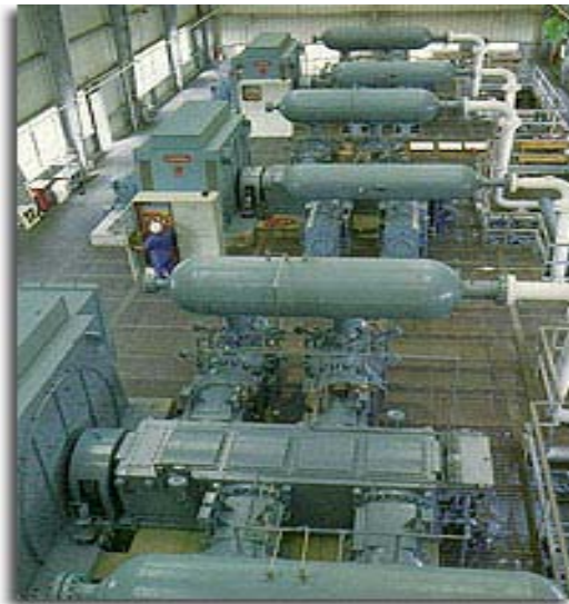
Three 8500 horsepower HHE-VL units compress natural gas to 2700 psi into underground storage caverns.
